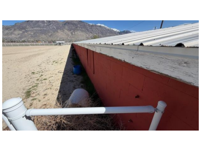
PHOTO 4: Red CMU walls and Red Wood Trim contain lead
